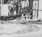
BLACK TYPON-BLOCK: Employees of an Aruba contractor raise a fire-wall tapon-block round a tank near the Lago Heiweg's lake.
